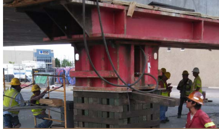
Inspecting the new bridge after raising it level with Pecos Street. (Photo courtesy of Rocksol Consulting Group.)
