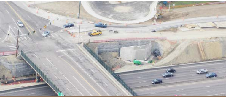
Aerial view of the old Pecos bridge prior to demolishing. (Photo courtesy of Kiewit Infrastructure.)
