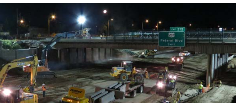
Night-time demolition of the Pecos bridge over I-70. (Photo courtesy of Wilson & Co.)
