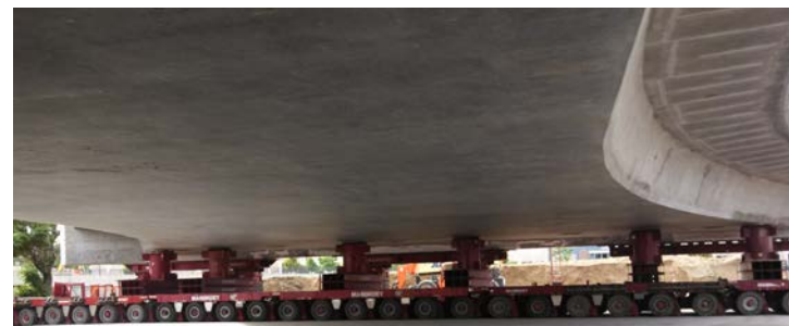
The new bridge, painstakingly transported into place, is jacked up flush with the Pecos Street surface. (Photo courtesy of Rocksol Consulting Group.)
