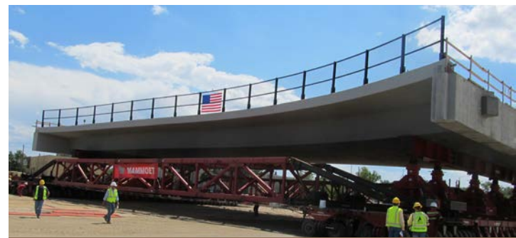
Slow movement of the pre-built Pecos bridge begins. (Photo courtesy of Colorado Department of Transportation.)
